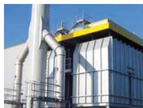
Exhaust gas purification via LARA®
