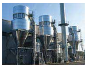
Dedusting of the machinery hall
